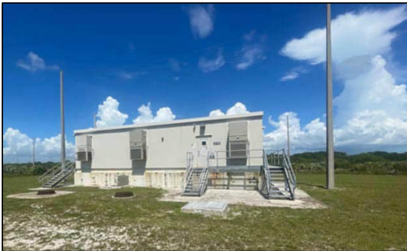
Photograph 4. Electrical Switch Station, Facility 38015, facing west.
