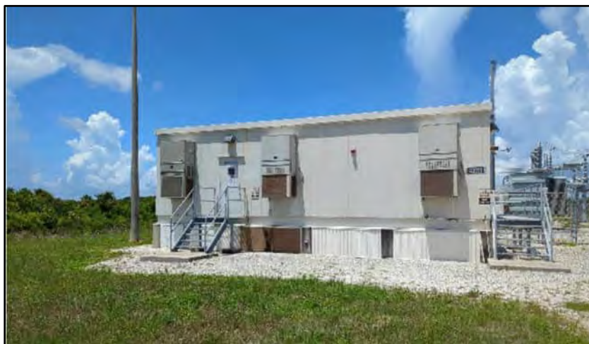
Photograph 13. Delta IV Power Control Center, Facility 43313 (previously unrecorded), facing west.
