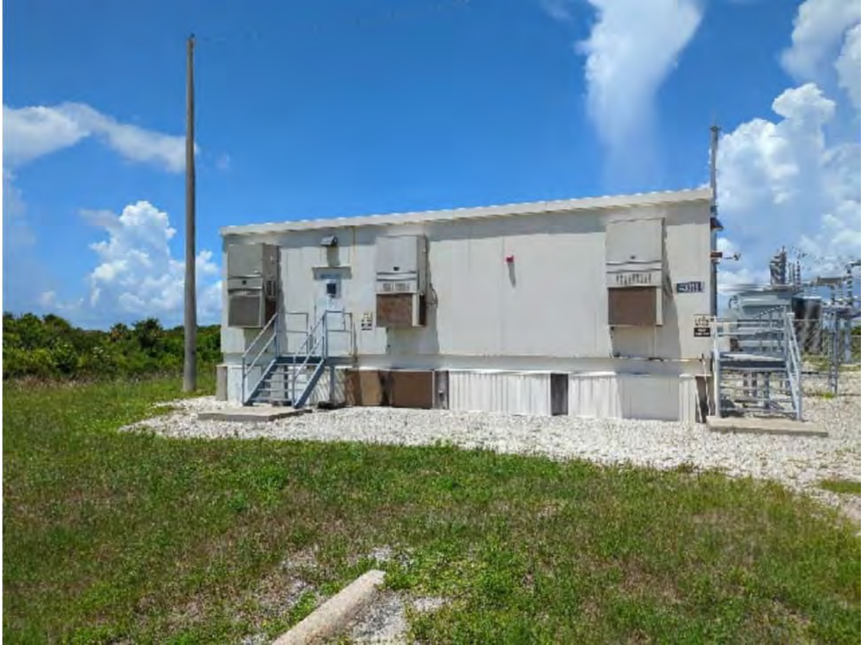
Photograph 1. Delta IV Power Control Center, Facility 43313 (previously unrecorded), with an electrical substation in the background, facing west.
